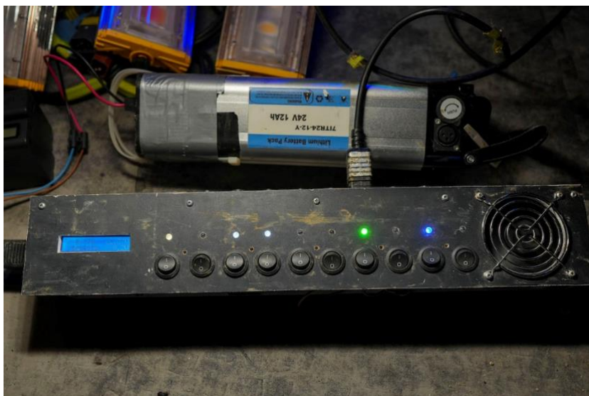
Switchbox. daz disley, 2023.
