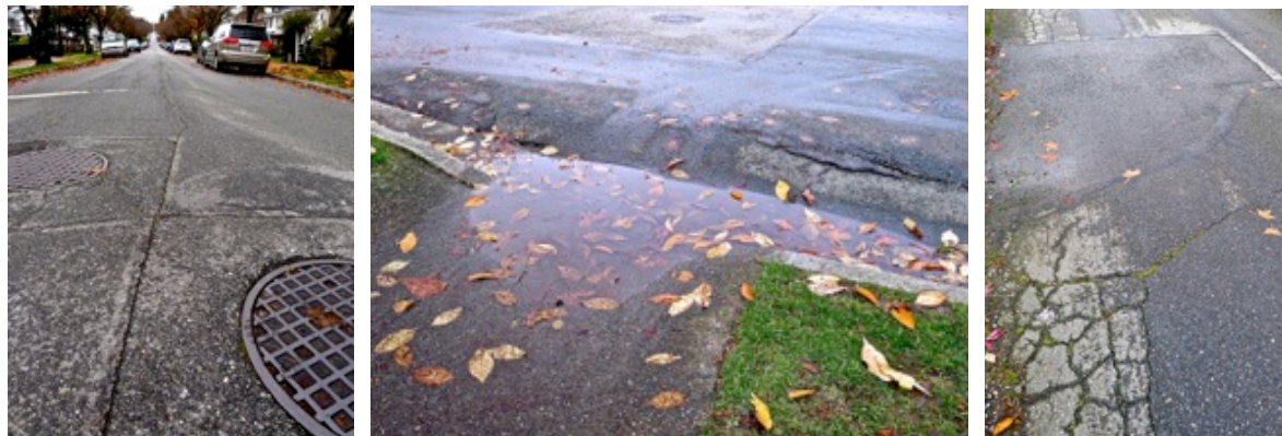
The state of the asphalt along a stretch of the site of act 2, “The Swamp.” Notice the buckles, bends, and cracks in the pavement as of November 2012. Photographs by author.
